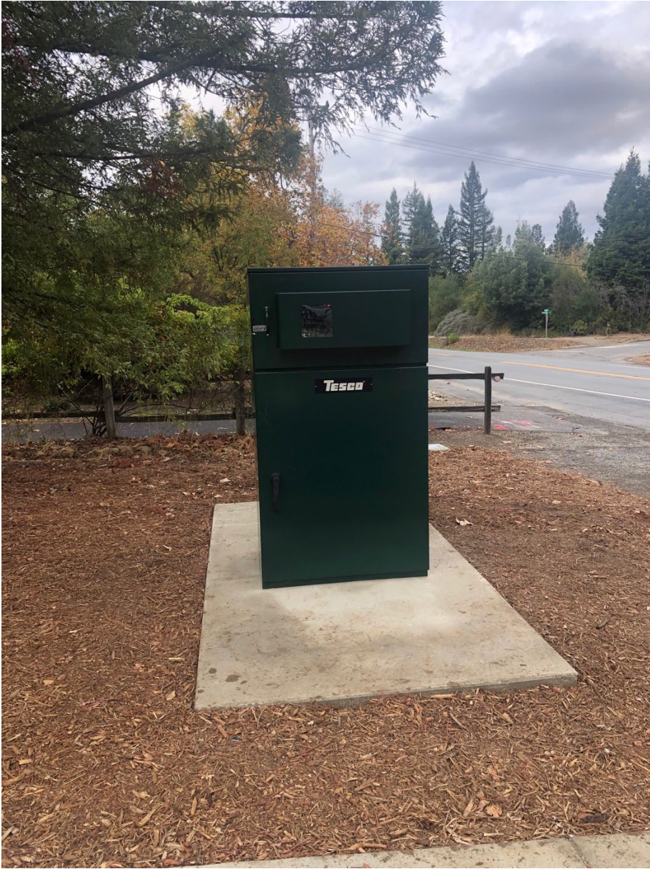
(Electrical cabinet Northeast corner Station 8)
