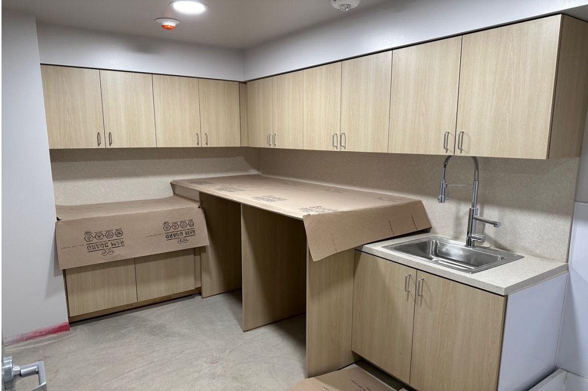
Second floor laundry room with casework and fixtures complete, awaiting washer/dryer units from interim station 7.
