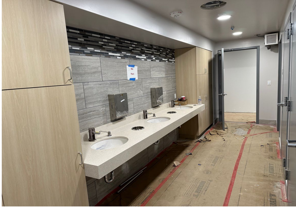
Downstairs bathroom, wall and floor tile complete, casework complete, fixtures installed, paint finished
